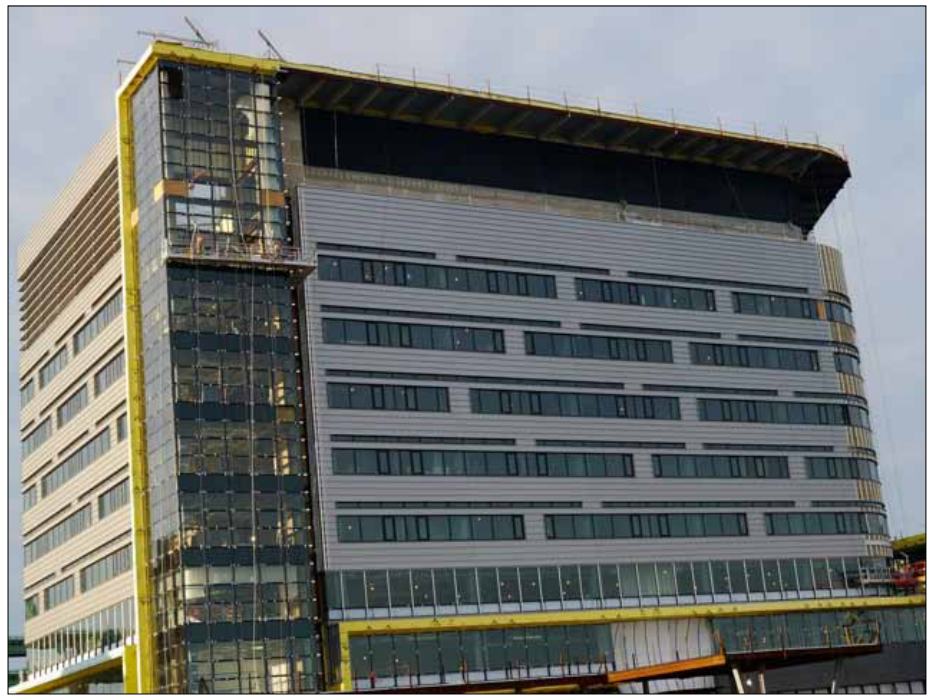
Spaulding Rehabilitation Hospital building was buttoned up in December, 15 months after breaking ground at Yard's End. Next year at this time, it will be preparing to open for patients.
