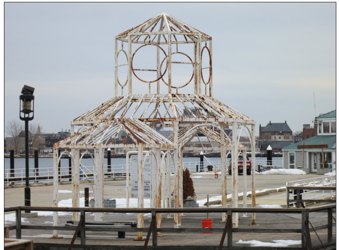
Gazebo on Pier 8 will be removed for repair of pilings underneath, repainted, and reinstalled as part of the repair project.
