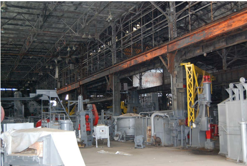
Interior View of Shed with Equipment
